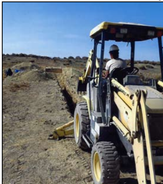
Figure 39. Trench A in the Main Quarry under excavation, October, 2021. Isaac Newton is the backhoe operator.
